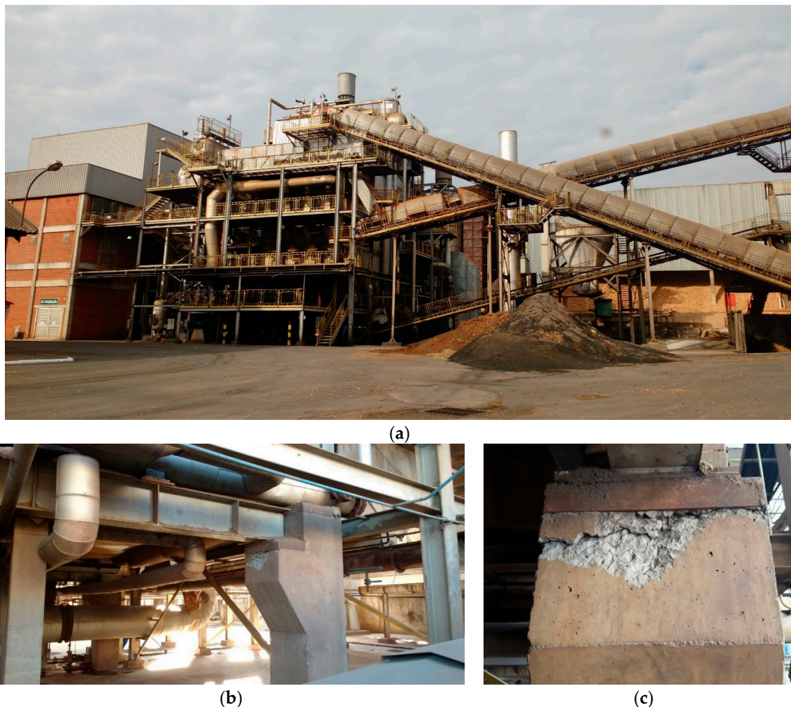
Figure 5. (a) Biomass industrial boiler; (b) reinforced concrete corbel supporting a W-beam; and (c) detail of the spalled concrete at the face of the corbel due to inadequate position of the load bearing plate.
