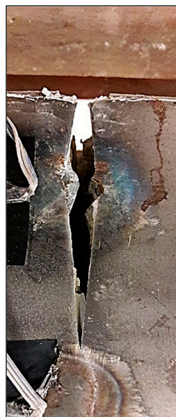
Figure 12. Steel rupture occurred at the bottom steel plate of the CC-W specimen.
