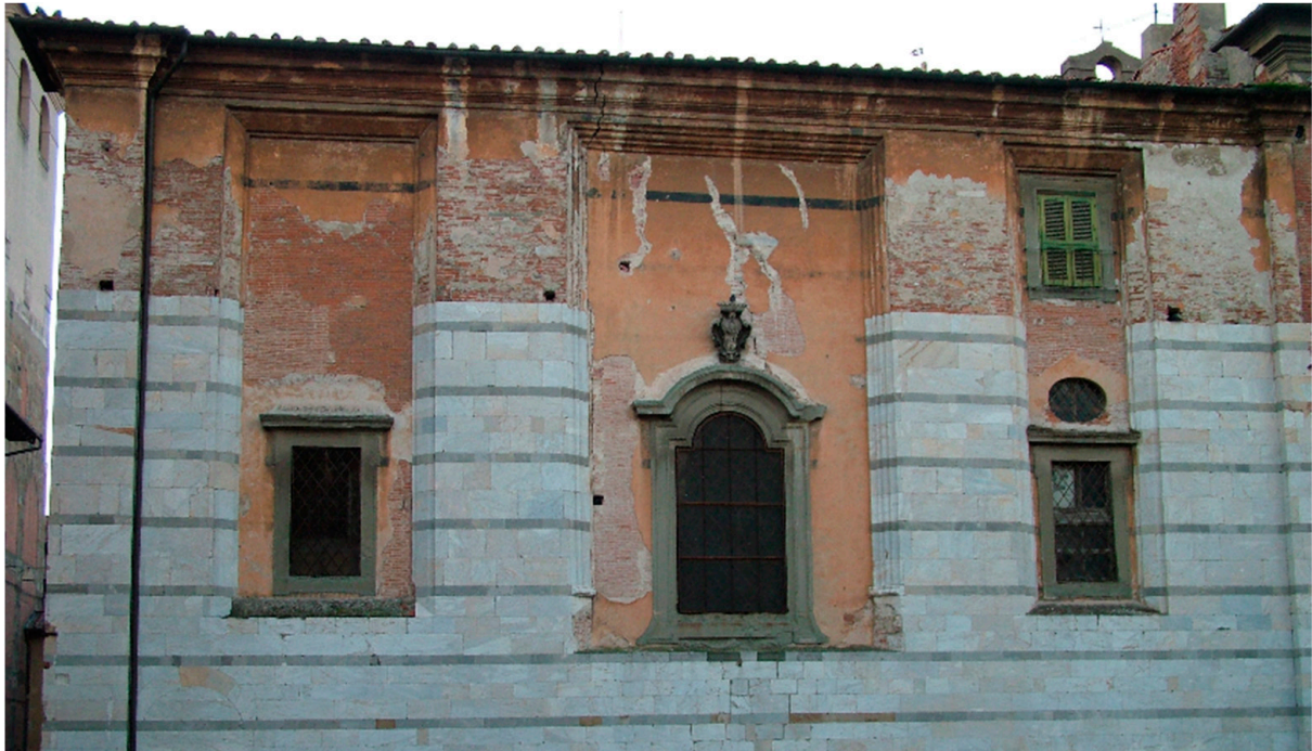
Figure 18. General view of the crack pattern on the rear façade.
