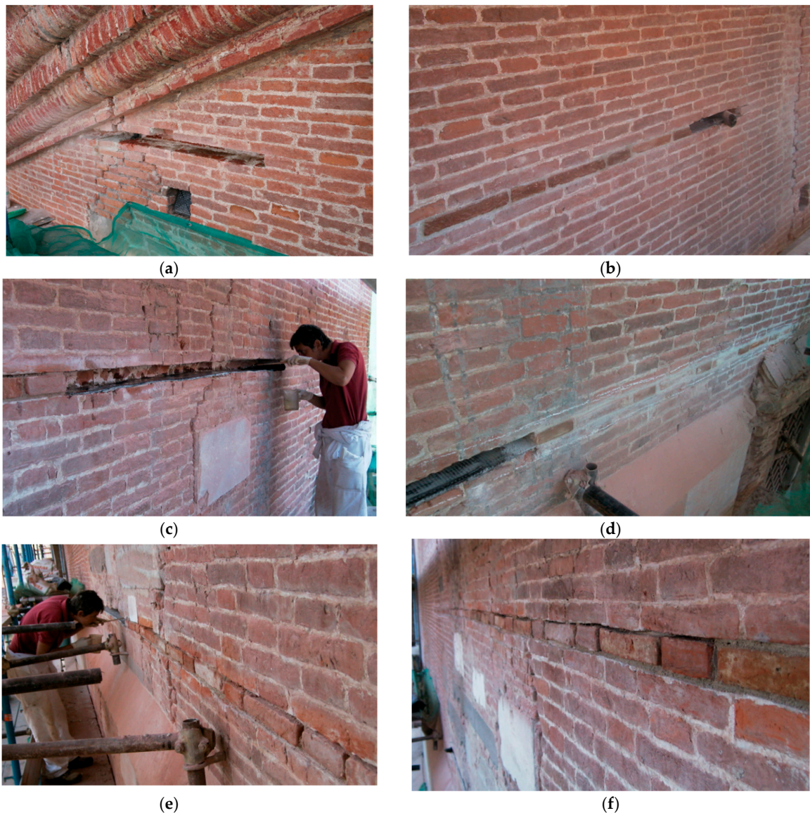
Figure 23. Relevant operational phases of the intervention: (a) removal of the first stretch of the brick course; (b) reconstruction of a stretch of the brick course, before unrolling the fiber roll; (c) unrolling and impregnation of fiber roll; (d) stretch of the brick course ready for reconstruction; (e) intervention in advanced stage; (f) intervention almost completed.
