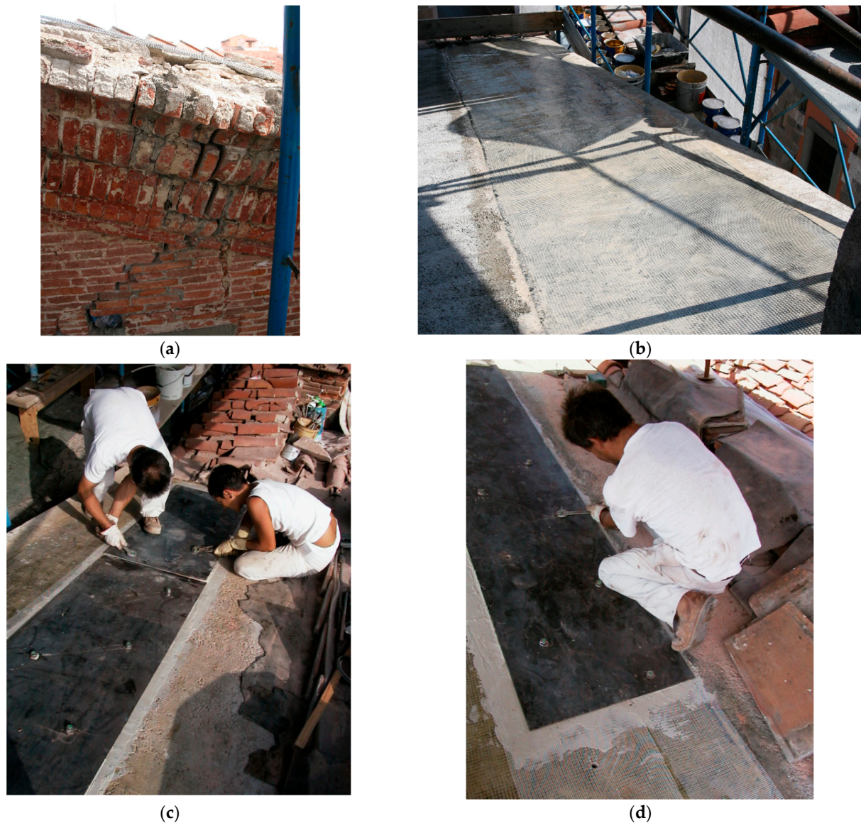
Figure 21. Phases of type A intervention: (a) edge joist before the intervention; (b) fixing of the carbon-fiber fabric; (c) upper steel plate; (d) glass-fiber net interposition for electrical insulation.
