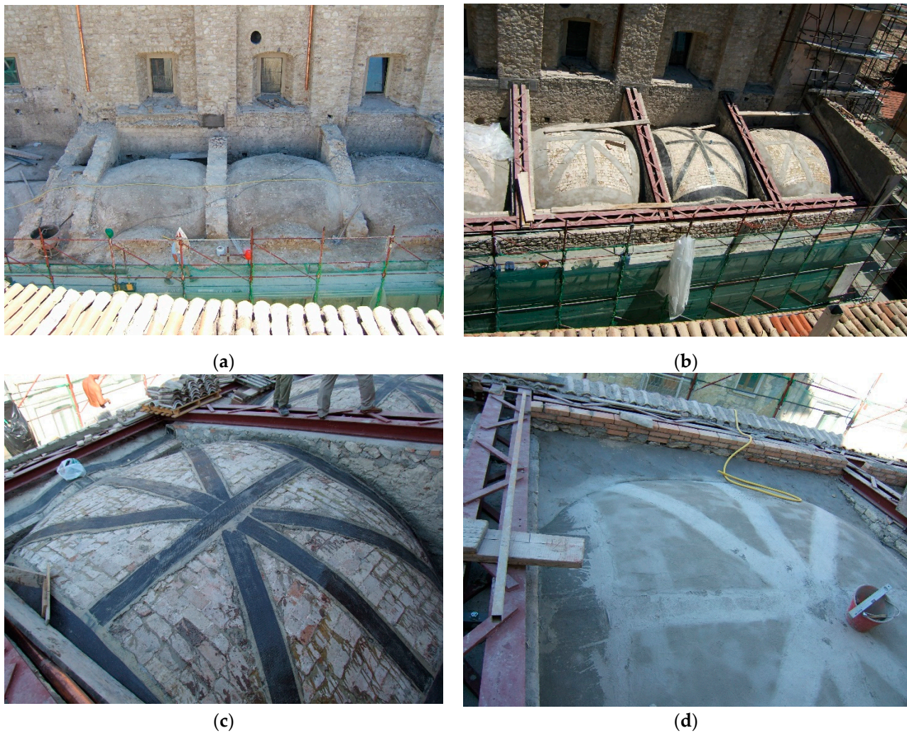
Figure 2. Composite strengthening of bohemian vaults with lunettes: (a) before the intervention; (b) application of composite strips; (c) detail of the composite reinforcement; (d) detail of the completed intervention.
