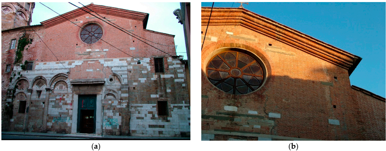
Figure 17. The crack pattern on the main façade: (a) general view; (b) detail.
