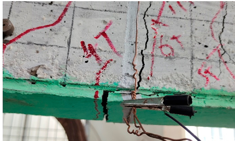
Figure 7. Failure modes of the smart mortar layer.
