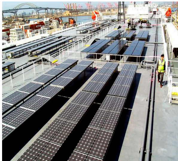
Figure 3. Installed solar panels, on Auriga Leader's deck [45], Reprint with the written permission from the photographer Tom Anderson 2019.
