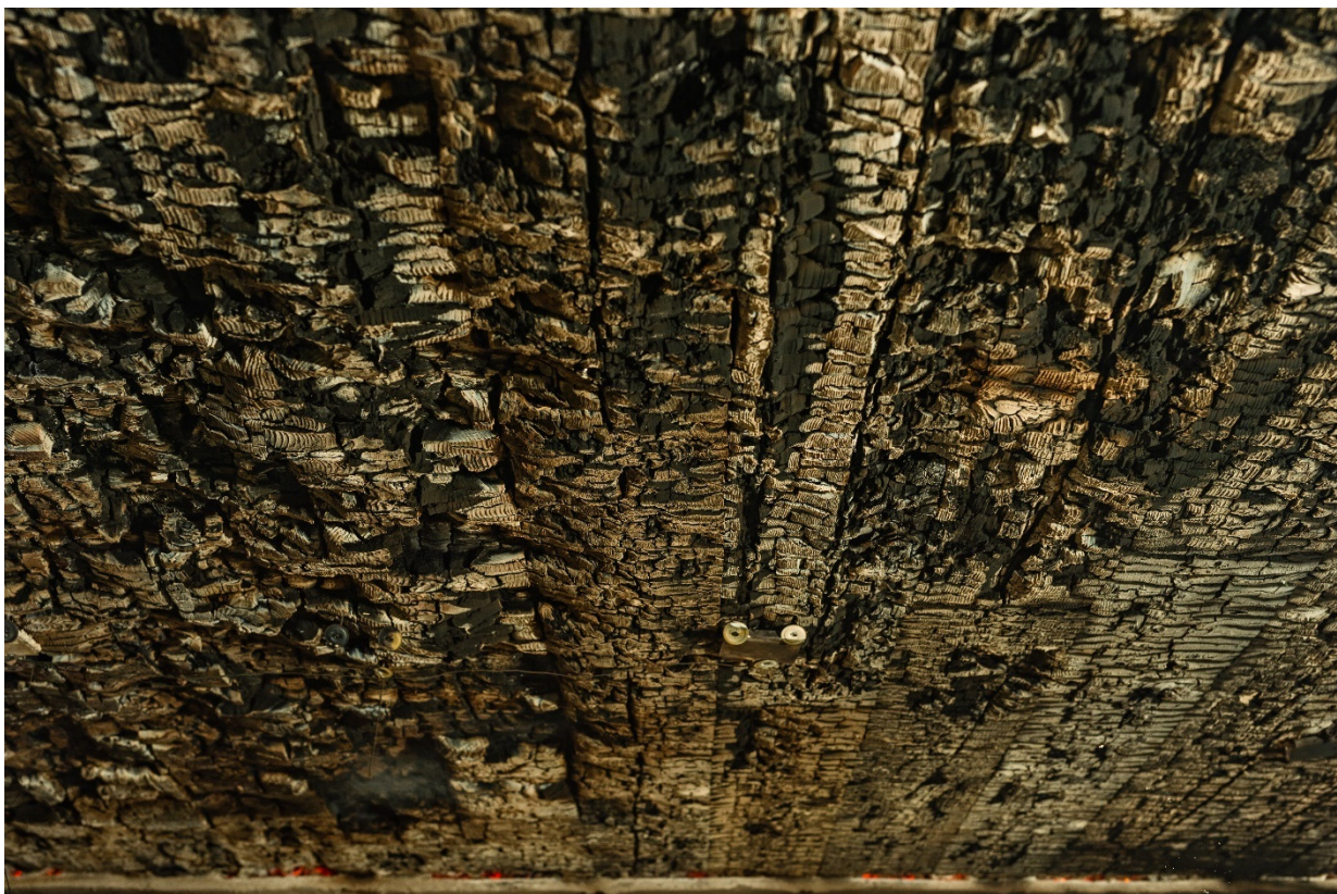
Figure 20. CLT soffit post-experiment in proximity to burner array in Experiment 3.
