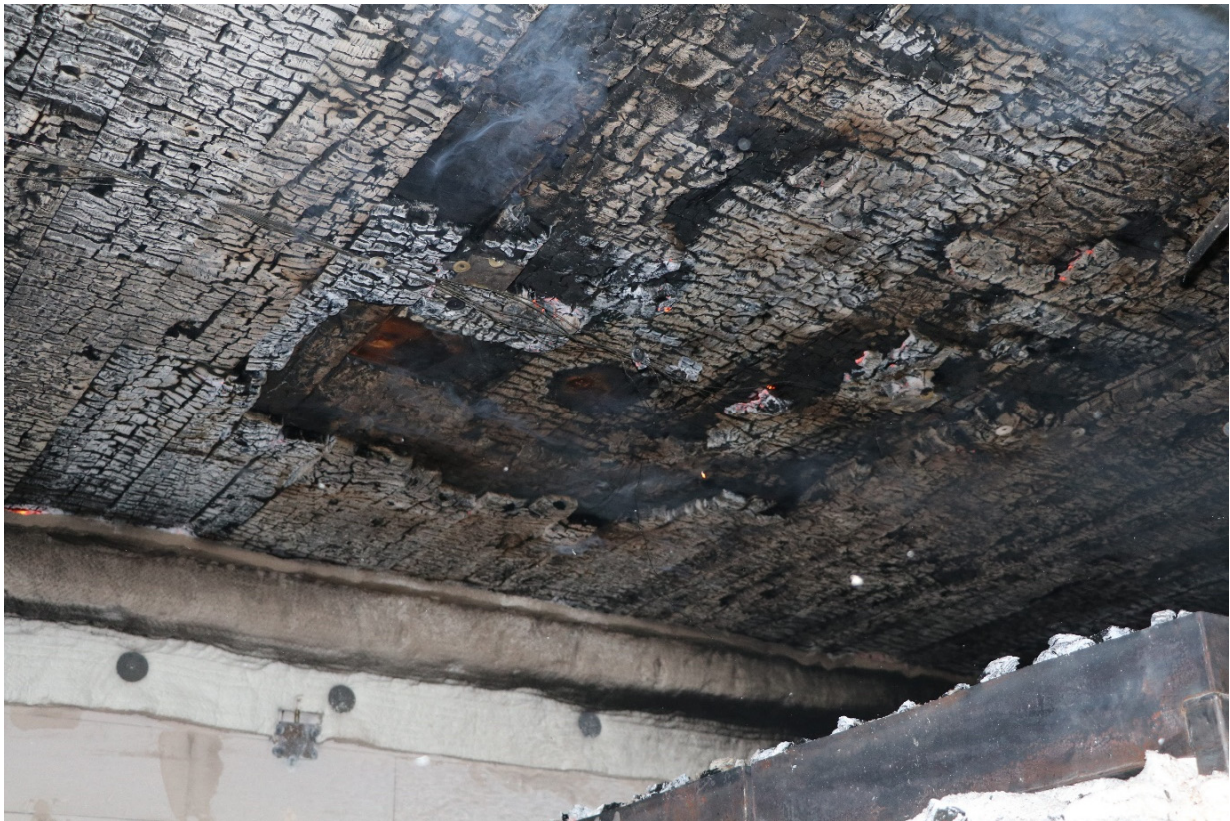
Figure 19. CLT soffit post-experiment in proximity to burner array in Experiment 2.
