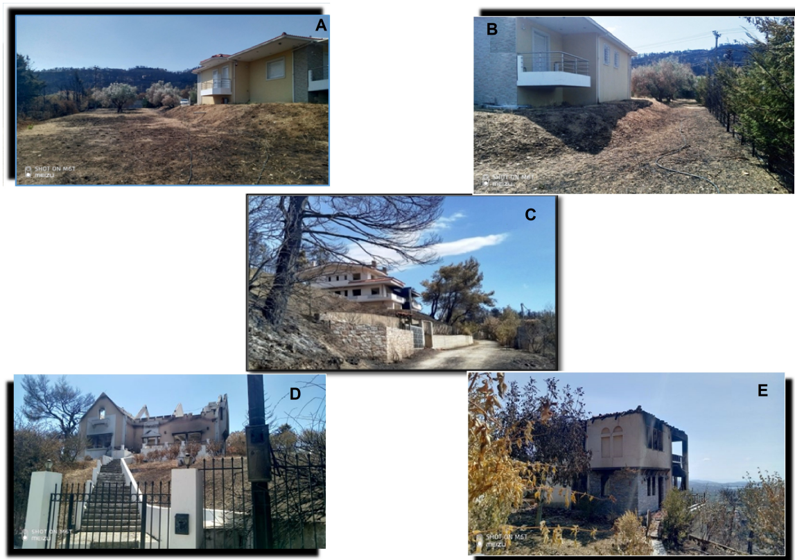
Figure 2. (A) Minor damage to a structure made of reinforced concrete, with double-glazed windows and aluminum shutters that were closed during the fire. The roof is tiled and there are no openings or gaps between the roof and the main building. (B) The vegetation at a zone of 10 m radius from the structure is <10 cm high without trees or shrubs. No damage occurred to the surroundings of the residence. (C) Moderate damage to the exterior of the structure (walls, shutters, etc.), without damage to the building itself. The reason for these damages is attributed to the existence of a pine tree at a distance <5 m from the building. (D,E) Major damages to the interior and exterior of the buildings. In both cases, trees were in contact with or within 2 m of the structure. Both structures are in steep ground inclination.
