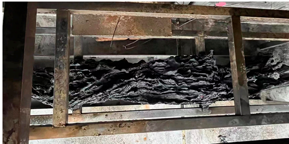
Figure 3. Photo of the charred cables.
