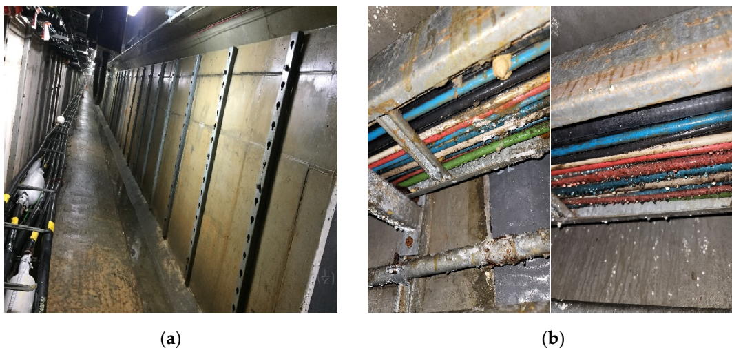
Figure 1. Condensation environment in underground utility tunnels (UUTs): (a) Condensation in UUTs; (b) Corrosion of cables and trays owing to condensation.
