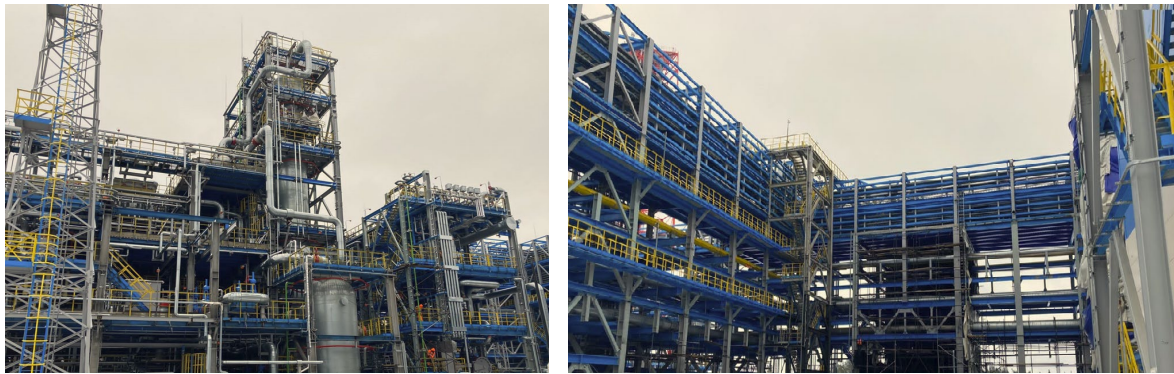
Figure 1. Platforms and trestles with structural fire protection at gas facilities. Author’s photo.
