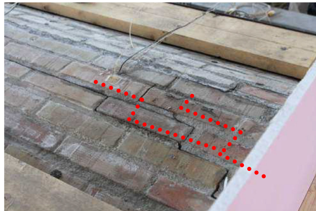
Figure 8. Crack pattern (red dot line) at the keystone in the experimental test.
