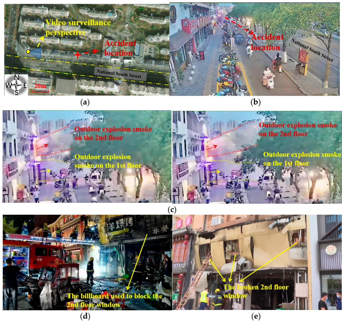
Figure 2. Peripheral pictures of the accident building: (a) accident spot; (b) video surveillance camera; (c) local magnification of the surveillance camera; (d) accident rescue scene; (e) accident scene after rescue.
