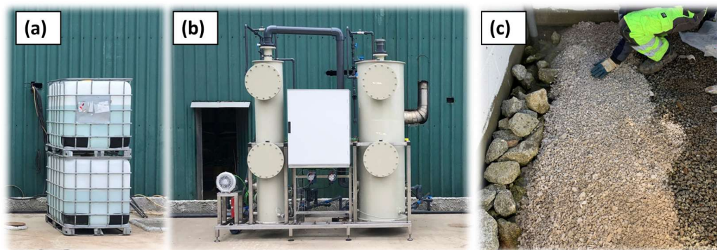
Figure 18. Pilot-plant: (a) tank (b) air stripping system (c) vertical wetland.
