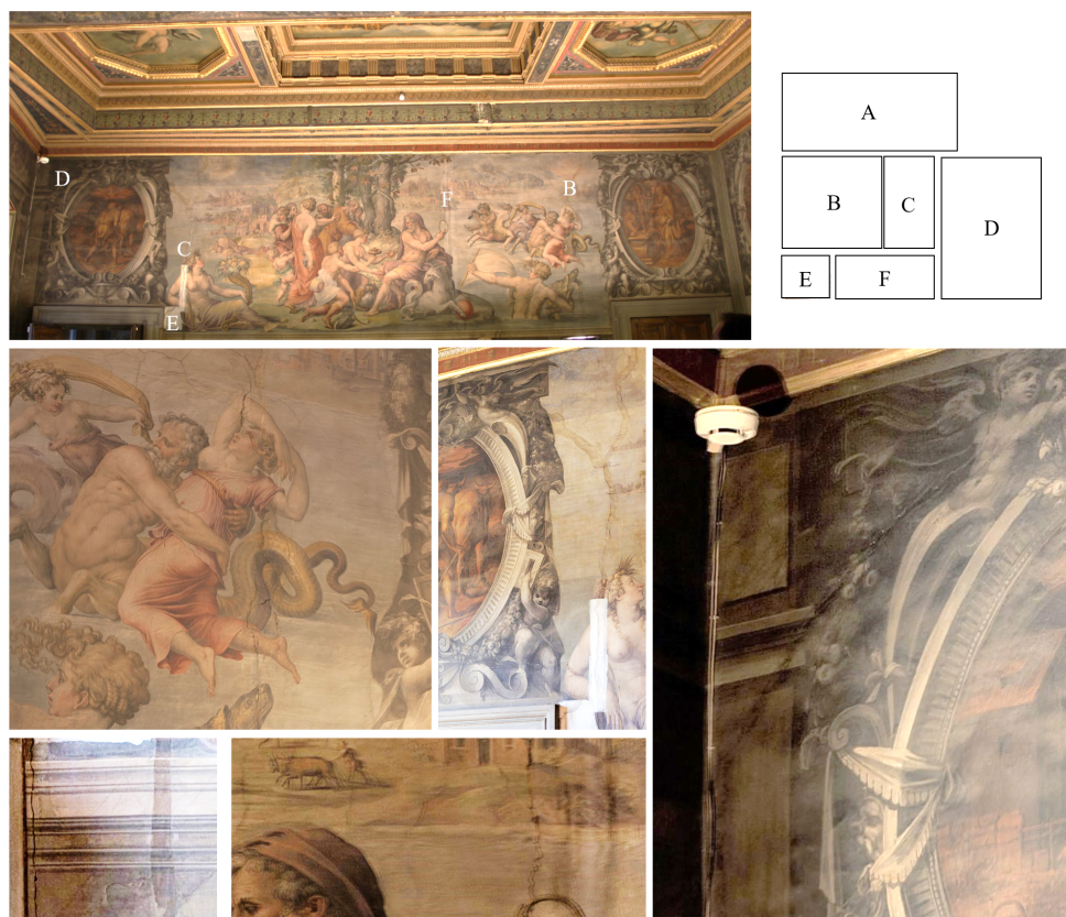
Figure 2. High resolution images of cracks in the Room of the Elements: (A) full illustration of western wall, (B–F) images of specific cracks on the western wall.
