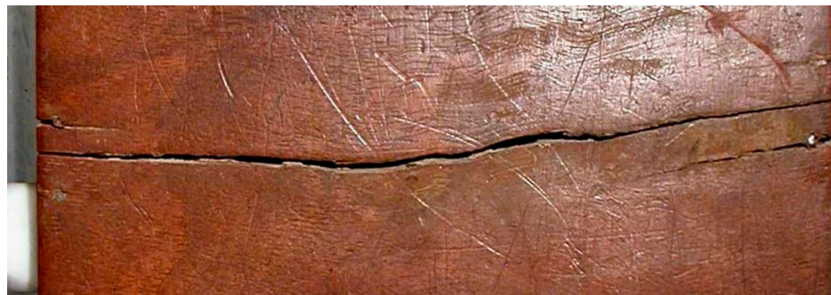
Figure 11. Detail of the outer side of the bottom. Irregular fissures—some of them favored by the insertions of “modern” nails.
