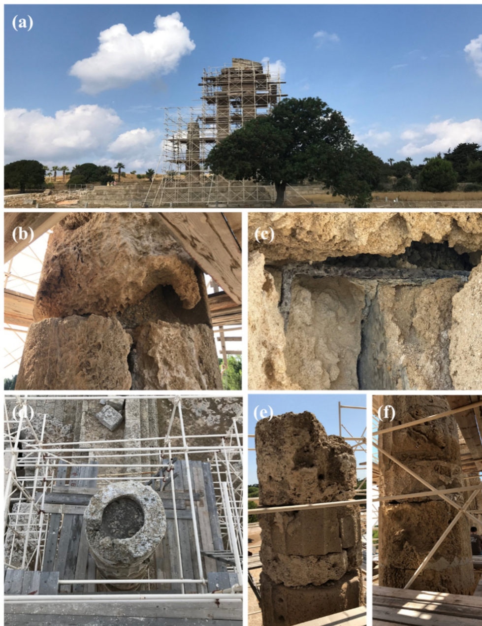
Figure 1. Temple of Apollo Pythios in Rhodes (a) Temple in its current state; (b) stone applied during the Italian restoration, in a bad state of preservation; (c) corroded metal element within column, disintegrated cement concrete and the deteriorated restoration stone applied during the Italian restoration; (d) image of free column from above, where one can notice how the interior of the column was carved out and filled with reinforced concrete during the Italian restoration; (e,f) upper and lower part of free standing column, where the manner in which the ancient, the restoration and the concrete materials have been used and bound together can be noticed.
