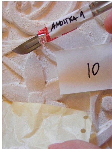
Figure 8. Sampling of surface salts (efflorescence).
