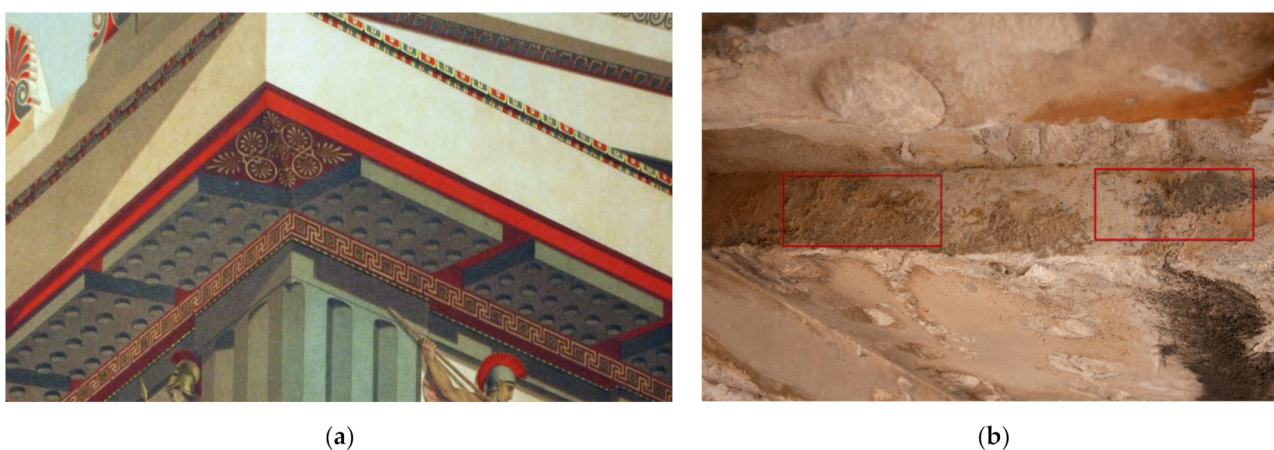
Figure 10. (a) Colour drawing of the cornice blocks dating from the 19th century (Fenger, pl.2, 1886) [45]. (b) The current state of the fourth west cornice block (north face). Black crusts and patina layers cover the surface of the mutule and viae. The guttae show severe damage and decay. Blue paint is visible in the areas where the crust has exfoliated (red frame).
