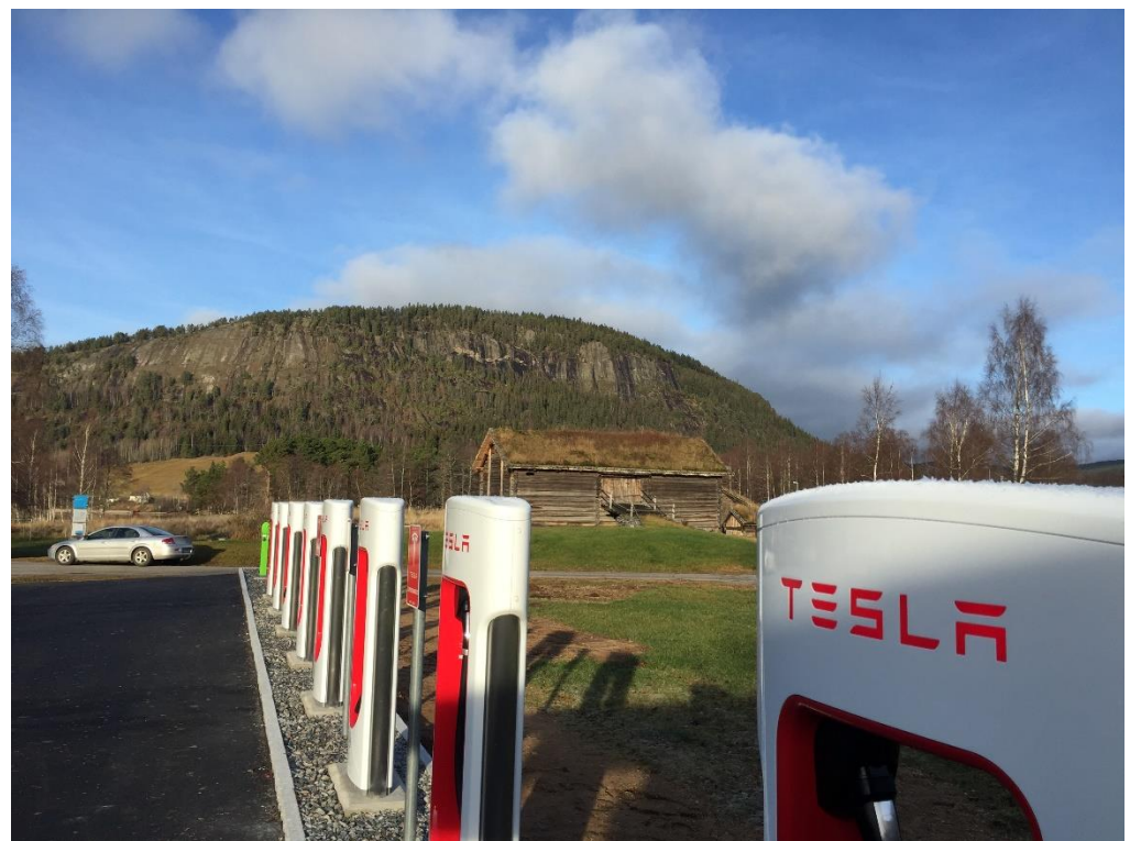
Figure 12. Charging stations in a row right in front of preserved built heritage at Bygland Bygdetun, Norway. Photo: Leira, for Visit Sørlandet.
