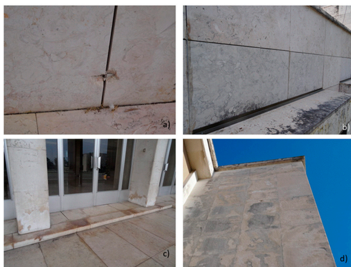
Figure 1. Examples of natural stone facade reactions to environmental conditions: (a) anchor rupture leading to strength loss; (b) biocolonization showing a relevant colour change; (c) white stains from saline efflorescence; (d) dark stains from water absorption, which might lead to slab detachment (photo credits: Vera Pires).
