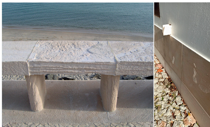
Figure 2. Examples of limestone elements subjected to natural salt weathering in a coastal area (photo credits: Joaquim Simão and Carla Lisci).
