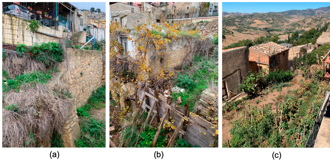
Figure 8. Partial demolition and securing along and between vico Vitale and via Riscato. (a,b) The downstream situation shows the provisional shoring and partial reconstruction of the retaining wall. (c) Upstream situation with the use of the infilled area as a private vegetable garden.
