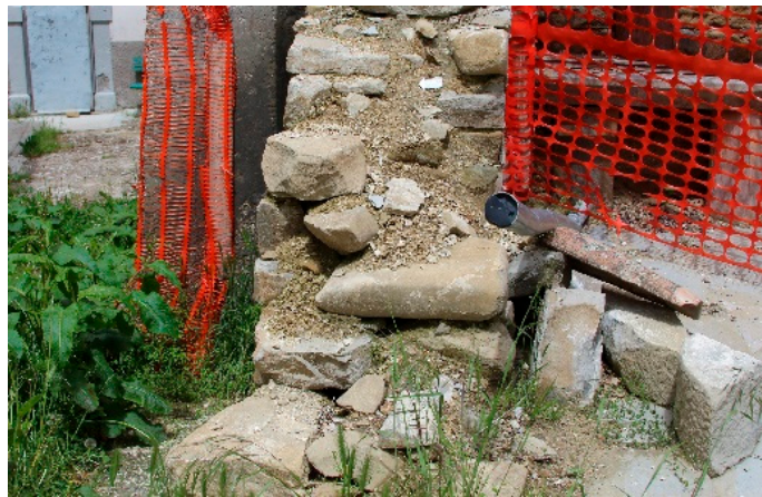
Figure 10. Wall section exposed following a collapse in Cornillo Nuovo, a hamlet of Amatrice (RI). Author photo.
