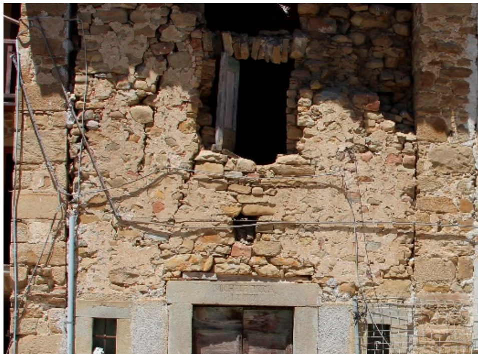
Figure 11. Building with traces of traditional plaster in Collocetra, a hamlet of Amatrice (RI). author Photo.
