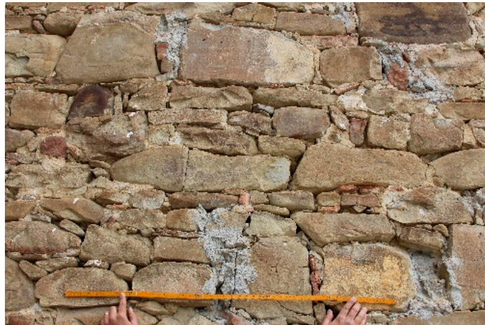
Figure 7. Typical wall texture of a historic building in the territory of Amatrice. Author photo, Cornillo Nuovo, Amatrice (RI).
