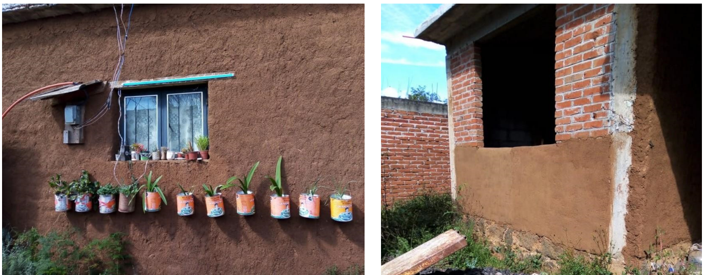
Figure 12. Final result of the earthen refurbishment after the rainy season. Source: A. Sanchez-Calvillo.
