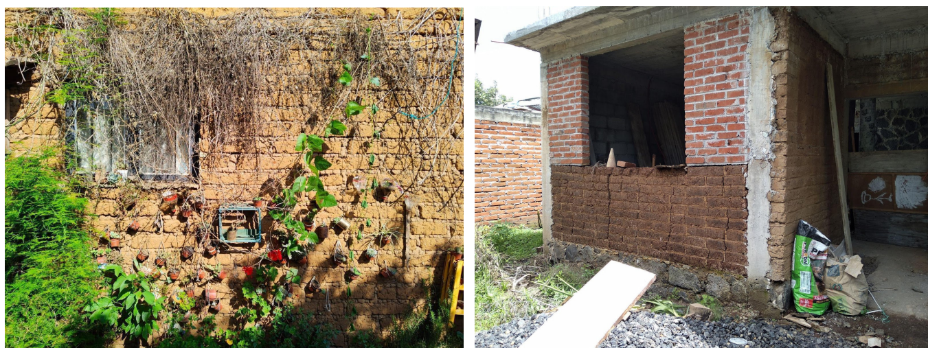
Figure 5. Adobe walls of Santa Anna Chapitiro before the intervention. Source: A. Navarro-Ezquerria.
