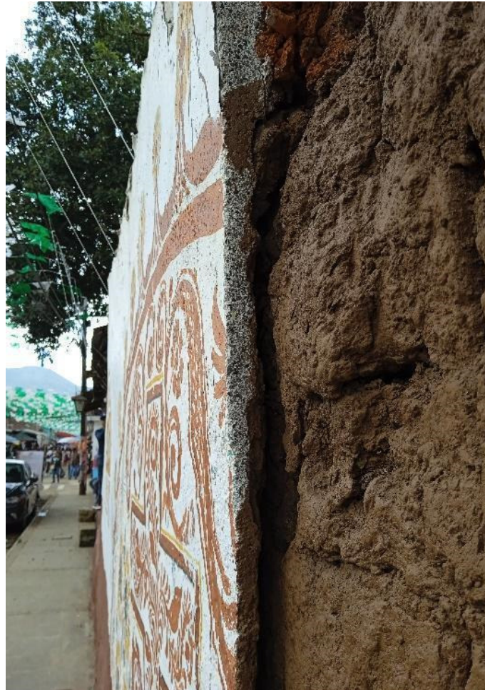
Figure 2. Pathology in traditional cladding on a historical building in Patzcuaro, Michoacan, Mexico. Source: B. González-Sánchez.
