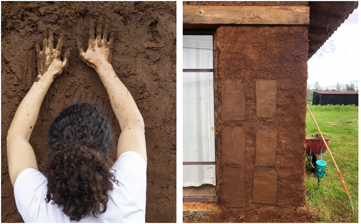
Figure 6. Testing mixtures by application on an adobe wall. Source: A. Solís-Sánchez and A. Navarro-Ezquerria.
