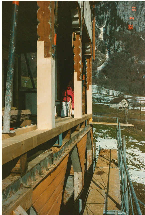
Figure 17. Walenstadtberg Housing. The repair of the pillars of the veranda by replacing the damaged parts. Material provided by Gody Kühnis.
