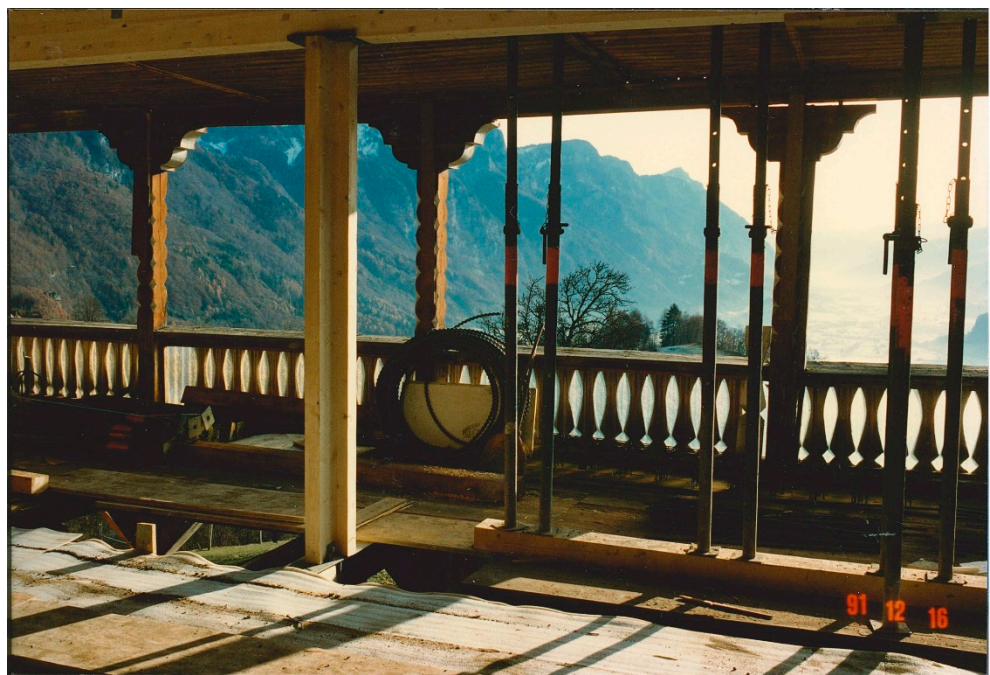
Figure 12. Walenstadtberg Housing under construction. Transverse continuity between the interior space and the veranda space. Note the Seesztal view from the veranda. Material provided by Gody Kühnis.
