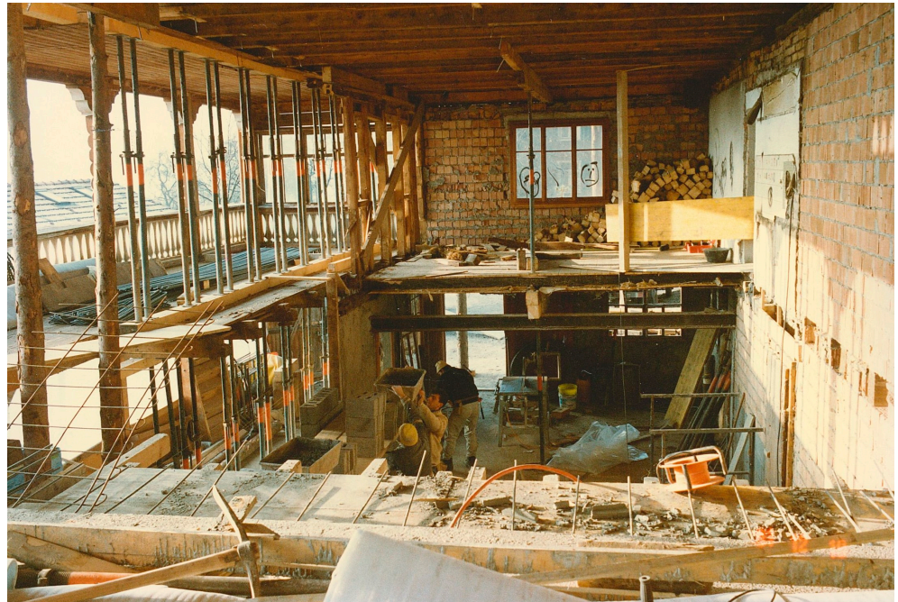
Figure 9. Walenstadtberg Housing under construction. Note the brick shell on the southwest and northwest façades of the ground and first floors. The new timber frame construction will be housed inside. Material provided by Gody Kühnis.
