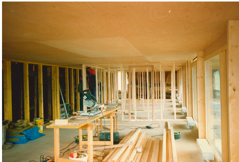
Figure 16. Walenstadtberg Housing under construction. Timber frame construction on the first floor. Material provided by Gody Kühnis.
