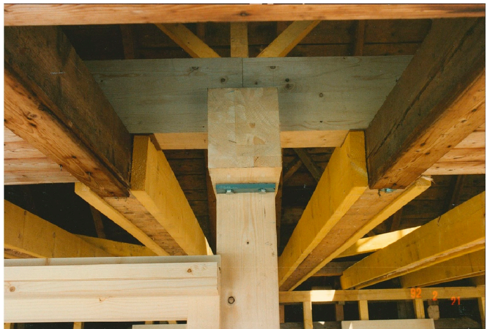
Figure 18. Walenstadtberg Housing. The reinforcement of the upper timber floor slab and fixing of the new pillars on the southwest façade. Material provided by Gody Kühnis.
