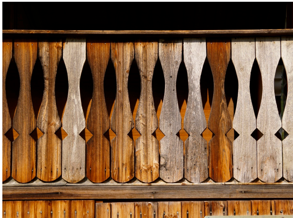
Figure 20. Walenstadtberg Housing. The restoration of the balustrade on the first floor by only replacing the damaged parts. Silvia Alonso.
