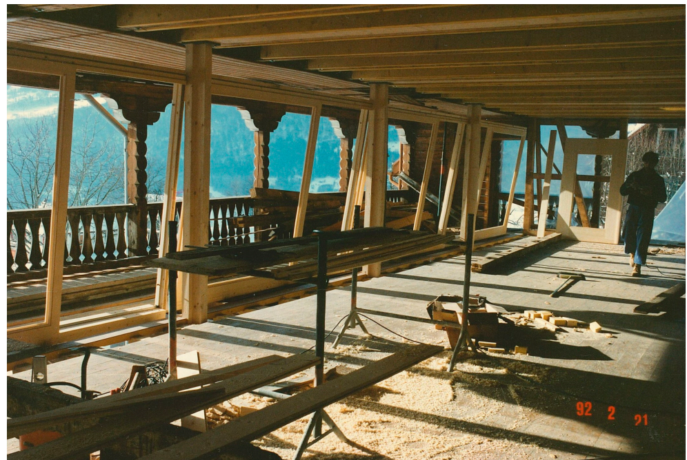
Figure 10. Walenstadtberg Housing under construction. The placing of the wooden windows between columns of what we have called the glazed loggia. Material provided by Gody Kühnis.
