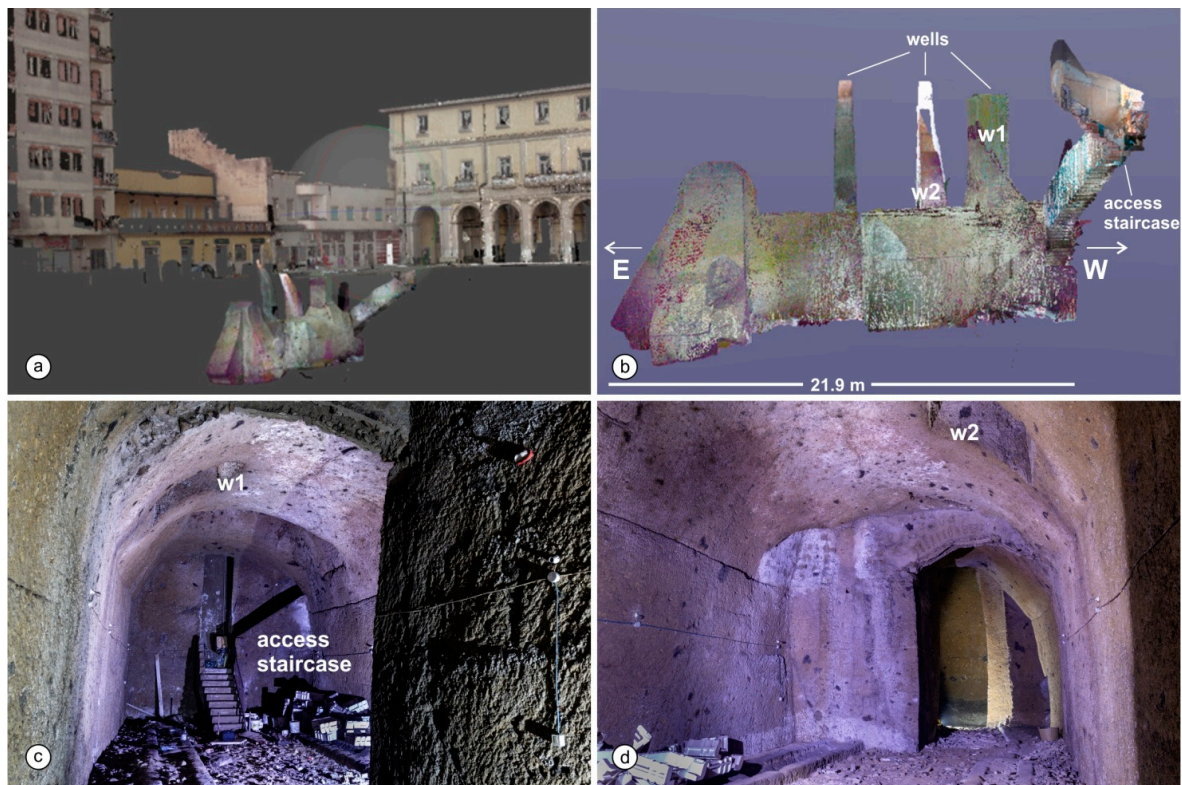
Figure 9. Representation of the cavity at the south-west edge of Piazza Municipio (a), through processing of the laser scanner survey. Note the position of the cavity with respect to the above buildings; (b) longitudinal section of the cavity; details of sector 1 (c) and sector 2 (d) described in the text (Ph. M. Vigliotti).
