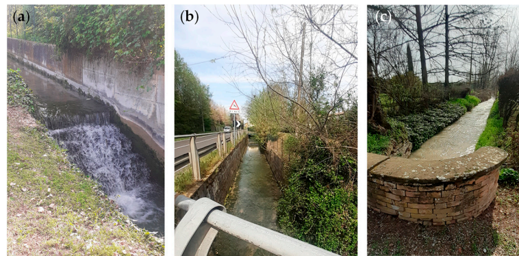
Figure 12. Exploitable sites along the canal for real field research applications: (a) bed drop, (b) embedded canal stretch, and (c) stretch suitable for real field hydrokinetic experimentation.
