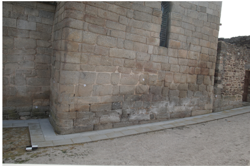
Figure 21. Pathology in north façade of the building.
