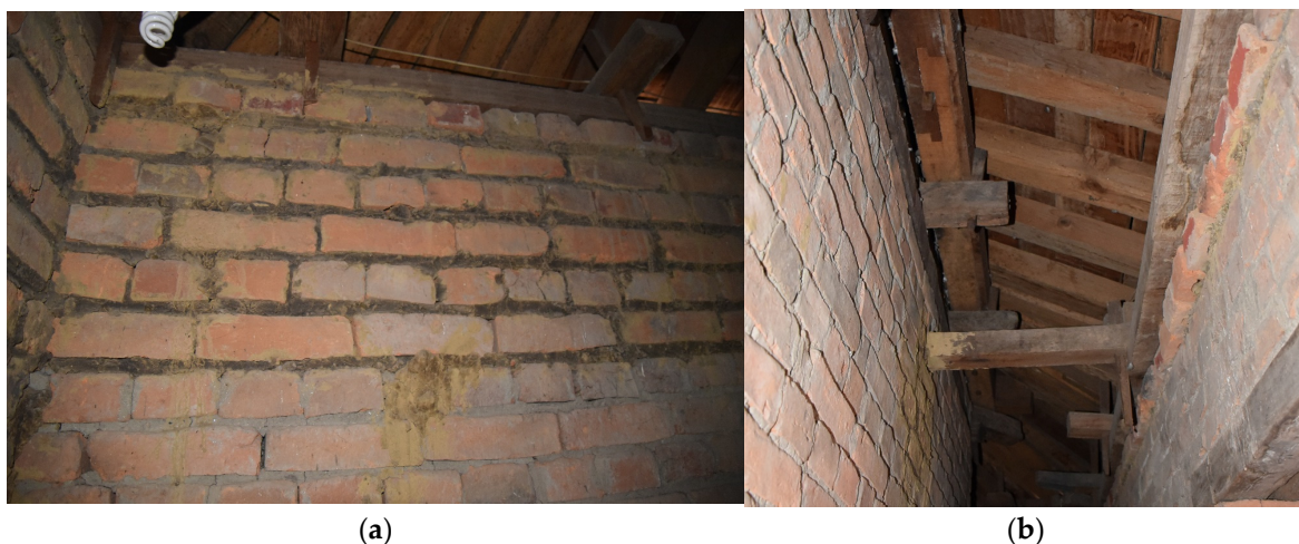
Figure 4. Exterior wall damages: (a) evidence of previous repairs; (b) relative out-of-plane displacement between upper timber crown beam and masonry wall.
