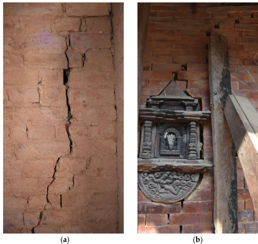
Figure 2. Shear cracks at ground level: (a) interior perspective; (b) exterior perspective.
