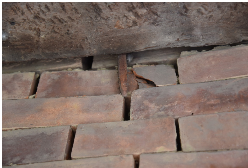
Figure 11. Broken bricks in contact area between peg and masonry wall at first-floor level.
