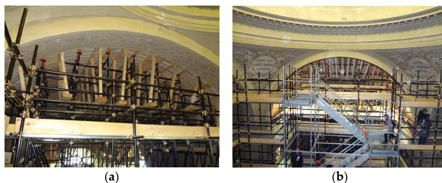
Figure 4. Church of Santa Maria Assunta in Reggiolo (RE, Italy): (a) Emergency scaffoldings to support the damaged vaults; (b) In situ inspection for executive design, using emergency scaffoldings. Photo credits: L. Ferrari, 2017.
