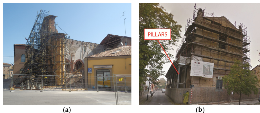
Figure 3. Structural scaffoldings in (a) Church of San Francesco d’Assisi in Mirandola (MO, Italy) and (b) Church of Beata Vergine del Rosario in Finale Emilia (MO, Italy). Photo credits: (a) MiC, (b) Google maps, 2016.
