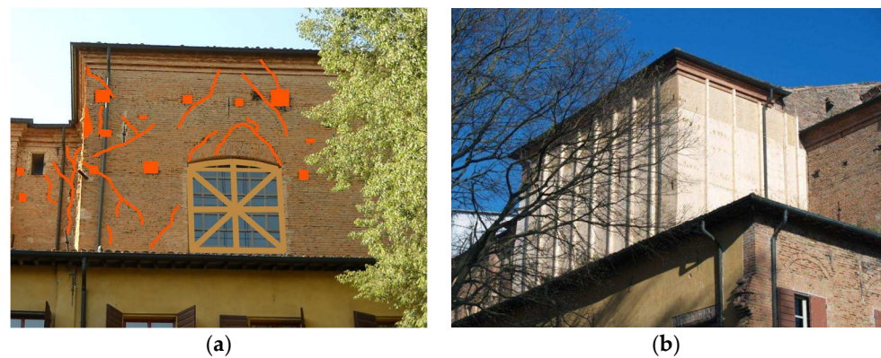
Figure 2. Transept of the Church of Jesus in Mirandola (MO, Italy). Crack pattern documentation (a) realized before the installation of the wooden confinement (b). Photo credits: Comune di Mirandola Provincia di Modena, Allegato 3 Scheda opera provvisoria urgente.
