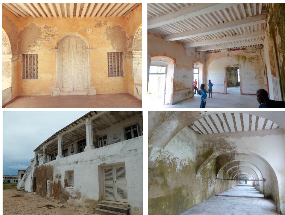
Figure 10. Some examples of the degradation phenomena (cracks, humidity areas, paint degradation, and weathering) observed in the Stone and Lime buildings. Reproduced with permission from Mariana Correia, author archive, 2018.
