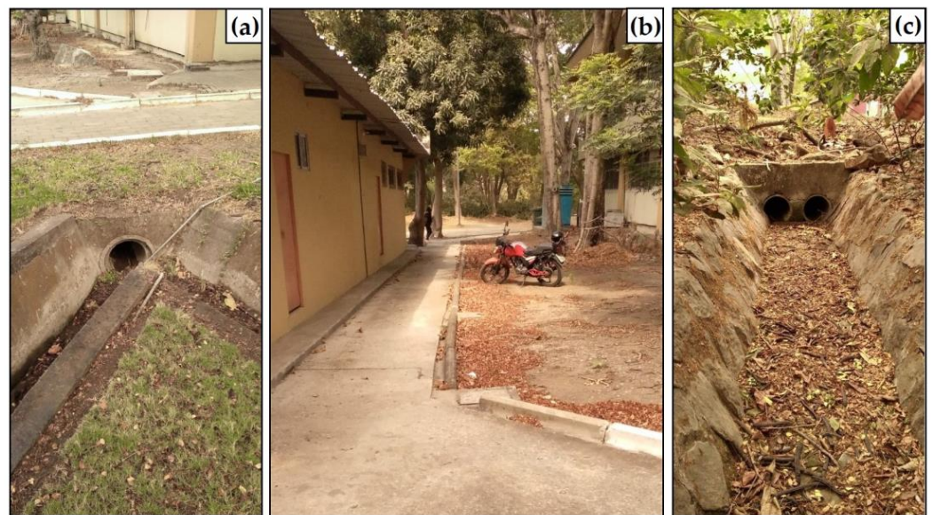
Figure 10. Point D analyzed: (a) pipe discharge into the canal; (b) stormwater inlet at point D; and (c) route of the stormwater collector.
