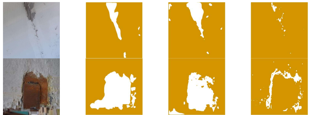
Figure 7. Representative test segmentation results for unseen category of steel corrosion.
