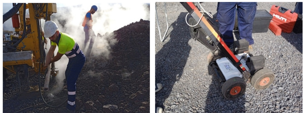
Figure 7. Borehole drilling in hot lavas, August 2022 (left), and Georadar survey to detect cavities, October 2022 (right).
