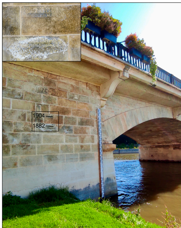
Figure 5. Limnometric scale and flood marks at the Palissy Bridge in Saintes.
