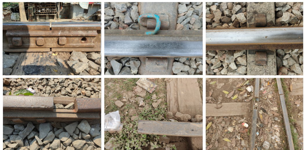
Figure 2. Samples of faults on railway tracks.
