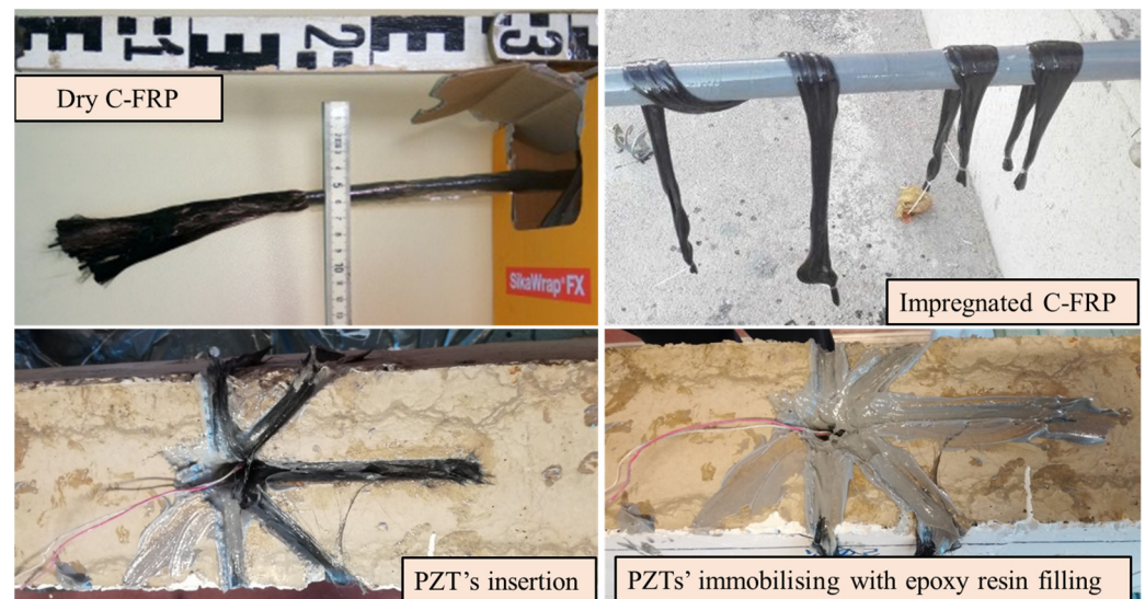
Figure 4. Insertion of the PZT transducers in the drilled holes assembled with the C-FRP ropes.
