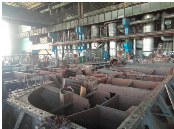
Figure 13. General view of the LPC (low-pressure cylinder) housing with the cover removed.
