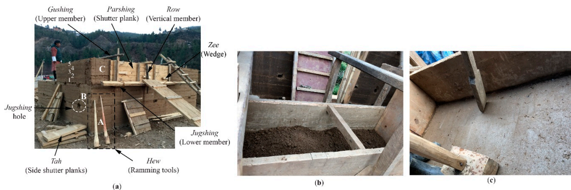
Figure 3. Construction details of U-RE specimen: (a) Rammed earth at third block showing formwork details, (b) Loose earth inside formwork before compaction, (c) Smooth and shiny finish after compaction.
