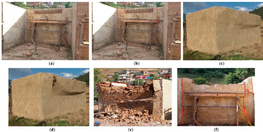
Figure 13. Failure mode of Mesh-RE: (a) crack initiation mesh plaster, (b) vertical cracks in mesh plaster, (c) bed joint crack in RE, (d) tearing of mesh, (e) and (f) final failure mode from the front and back view, respectively.
