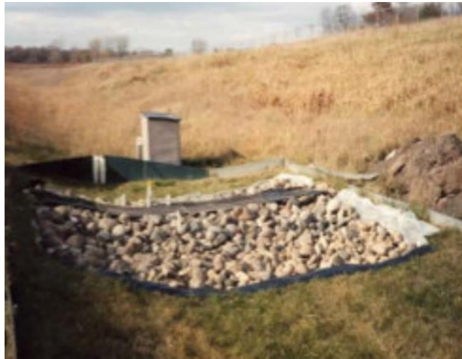
Figure 6. Pollution control research showing the check dam at MnROAD [5].
