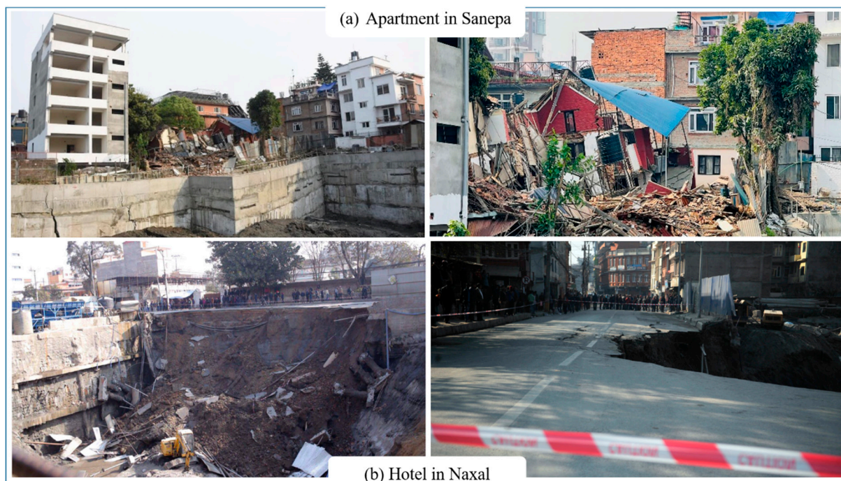
Figure 1. Failures in nearby structures: (a) Sanepa [4]; (b) Naxal, Kathmandu [5], during foundation excavation.
