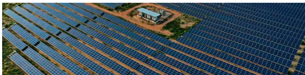
Figure 10. Bhadla solar park in India [20].
