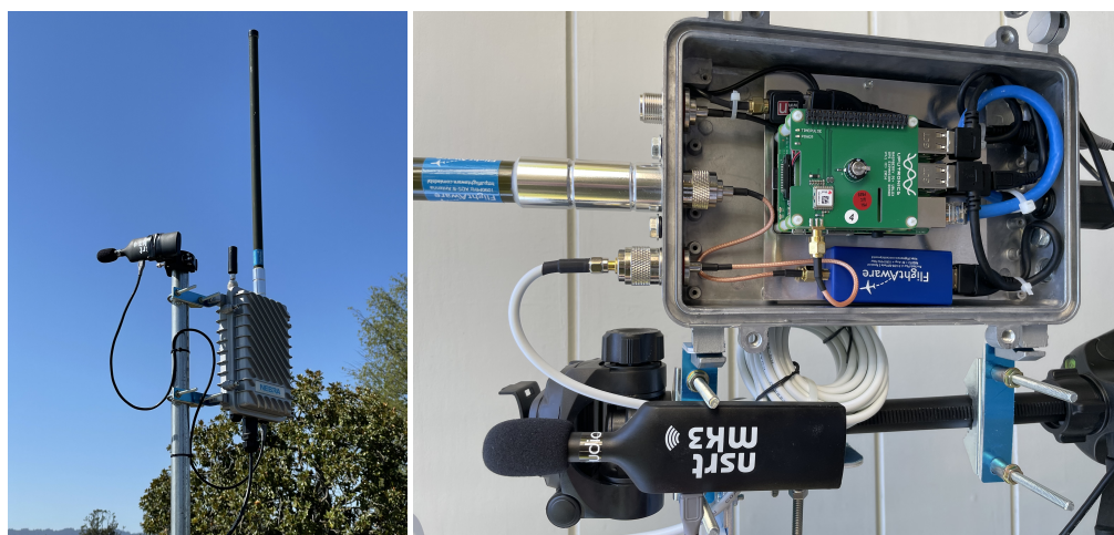
Figure 1. Sensor controller rooftop deployment with ADS-B and SLM (left), Sensor controller components (right).
