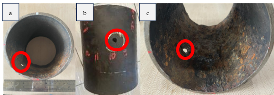
Figure 7. Pipe hole position (in red circle) after cleaning deposits. (a) View of the hole from inside the pipe; (b) view of the hole from outside the pipe; (c) Detail a.
