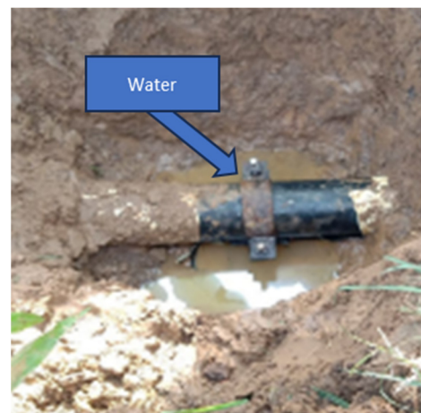
Figure 2. Water out of the leak.
