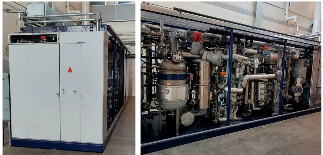
Figure 4. Hydrogen demonstration pilot plant. On the left is a side view of the hydrogen demonstration plant, and on the right is the front view of the hydrogen demonstration plant.
