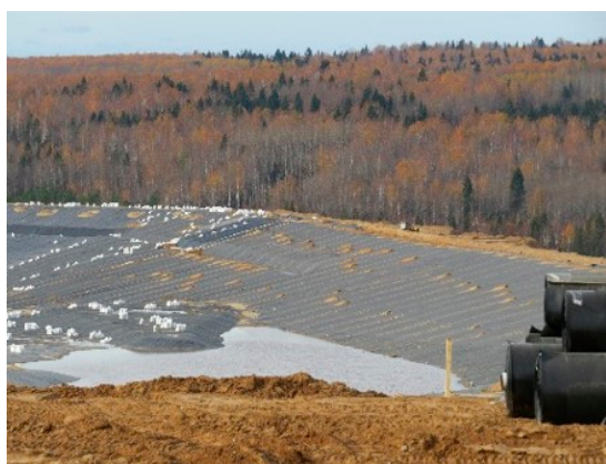
Figure 6. Use a geomembrane in new tailing slurry facility of potash mine at the Verkhnekamskoe deposit (Balakhontsevsky mining site).
