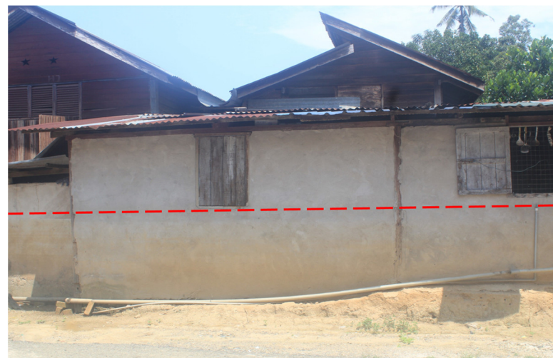
Figure 4. Flow water level during a flood (red line).
