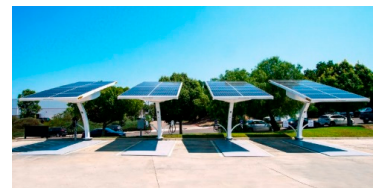
Solar Transportation—EV Infrastructure
