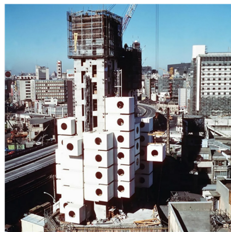
Figure 11. The promise of future replaceability remained fulfilled in Kisho Kurokawa’s Nakagin Capsule Tower, Tokyo, Japan, 1972 (image source: Public Domain).
