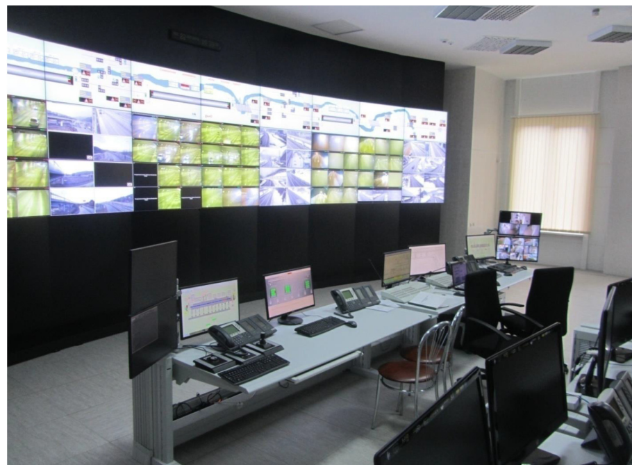
Figure 5. The dispatch control panel at ‘Olympic’ tunnels (Sochi, North Caucasus): location of a separate workstation for geotechnical monitoring in the control room; for each sensor, one can display a graph of its readings for the entire measurement time or for a certain period. The color scale (green-yellow-red) conveys the current state of the tunnel section in accordance with the selected threshold levels.
