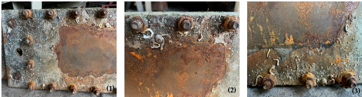
Figure 11. Photographic record obtained from the different zones identified in Figure 10, where it is possible to see in some detail (1) reduction of thickness after exposure; (2) degradation observed near an end containing screws; and (3) degradation observed near the opposite zone 2.
